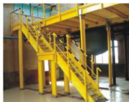
FRP platform & handrail
